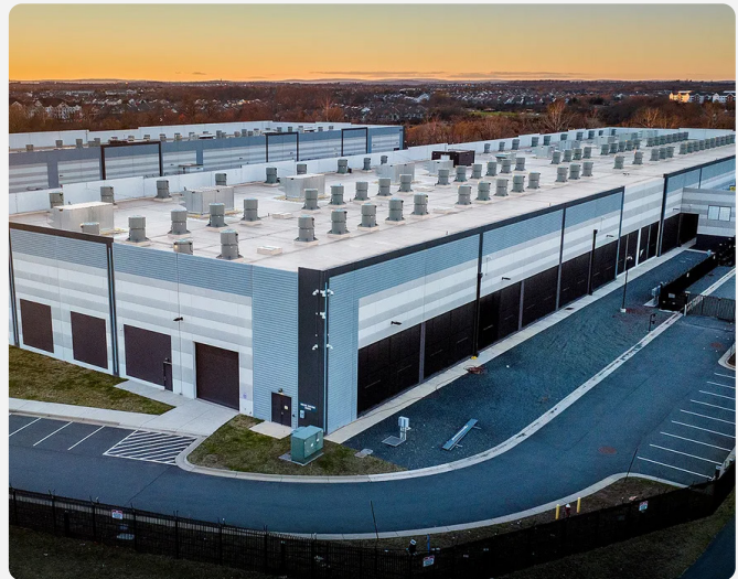
Amazon Data Center (Richmond County, Virginia)
